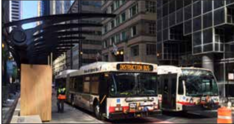
Construction to create distinct bus lanes, raised bus station platforms and more was ongoing in 2015 in downtown Chicago.
