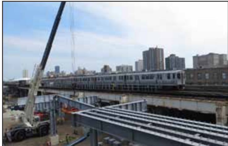
New track structure being installed near the Wilson Red Line station. The new 2,200 feet of elevated tracks will eliminate slow zones and improve service.
