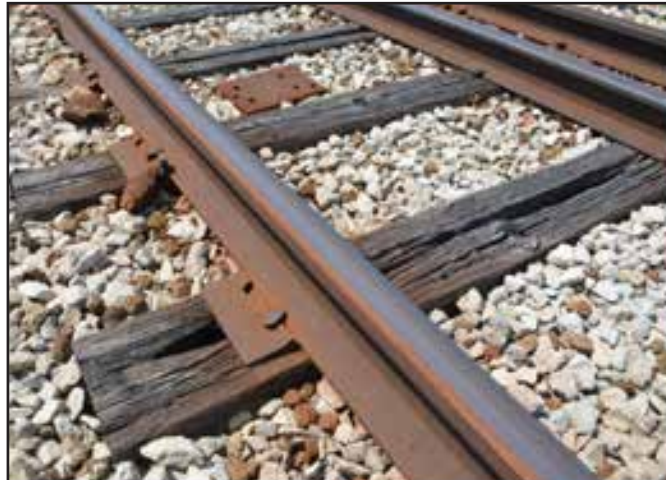
One of the main components of the Purple Express Improvement Project is to replace aging track ties that currently require trains to operate through slow zones in order to maintain safety for customers.
